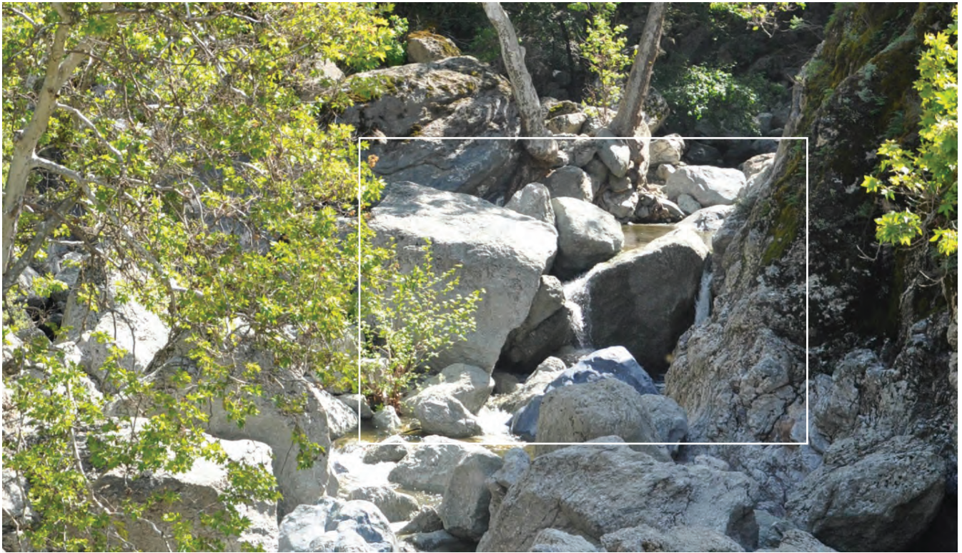
1. Existing View of Feature 10 Boulder Cut and Step Weir A site, looking upstream.
