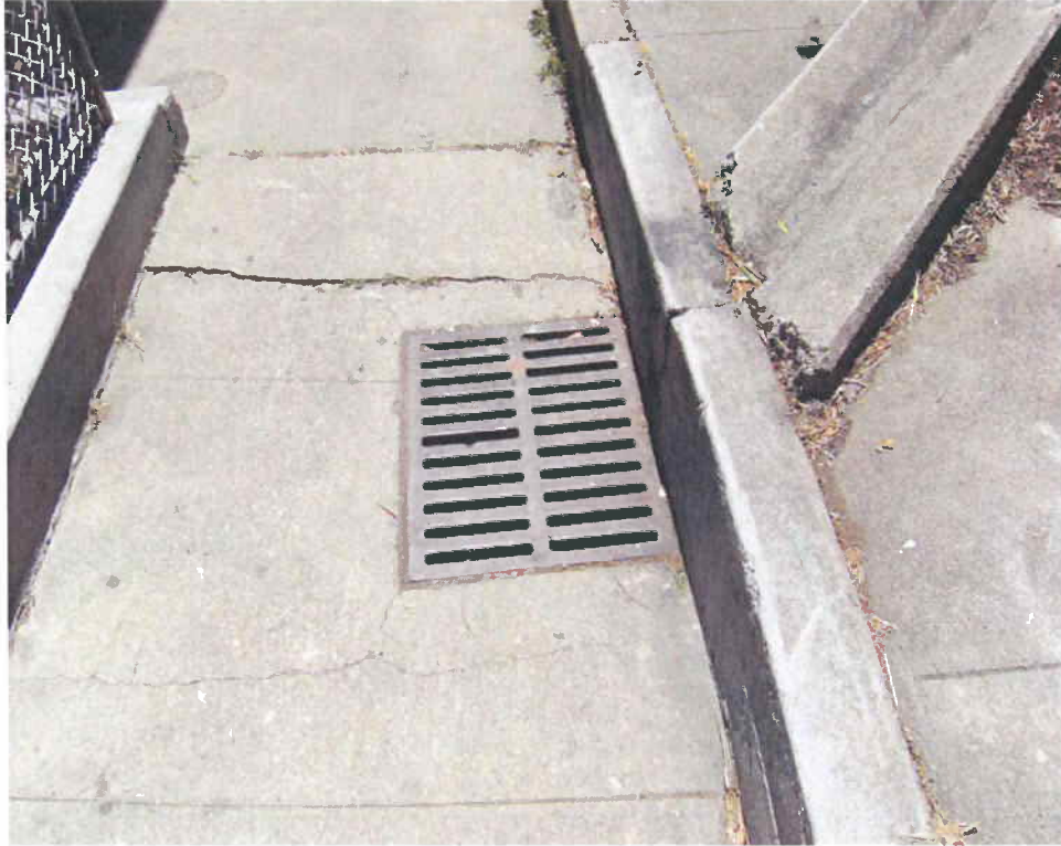
1) View of storm drain observed at the southwest area of the Site.
