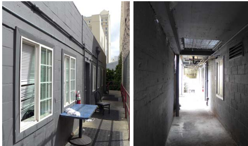
Figures 25 and 26. The south elevation of 530-532 Jones Street: upper level (left) and basement level (right).
