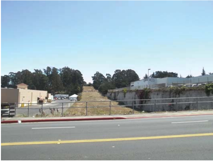
View 1: View to the south from Serramonte Boulevard to the construction zone in the SFPUC ROW
