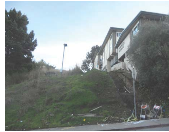
View 3: View to the south from Whitman Way to the construction zone in the SFPUC ROW, with the Park Plaza Apartments to the west
