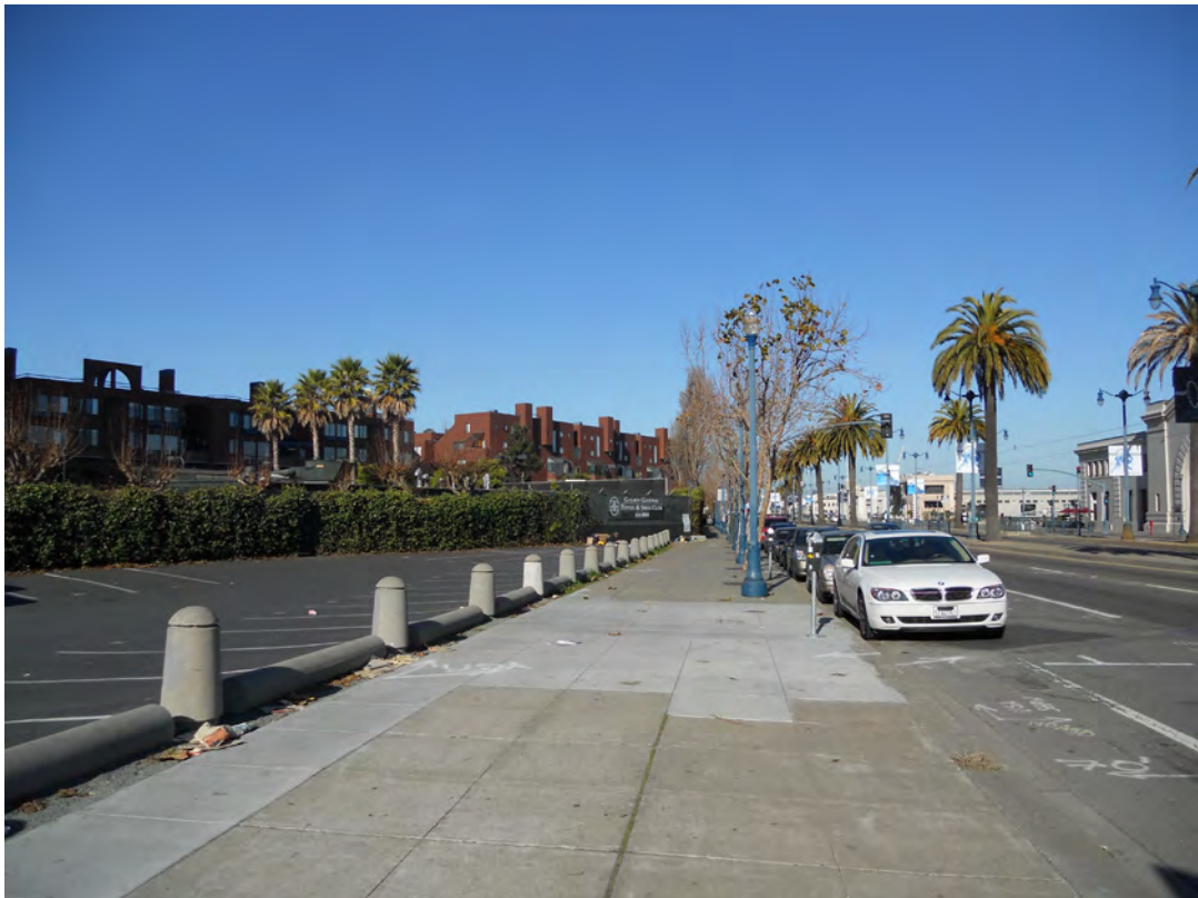
Photo 4: Northwest facing view of the vault construction work area from the southbound side of The Embarcadero.
